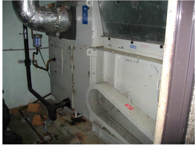
Typical air handler in mechanical room
