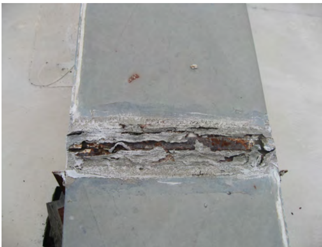
Typical deteriorating rooftop ductwork seam sealant
