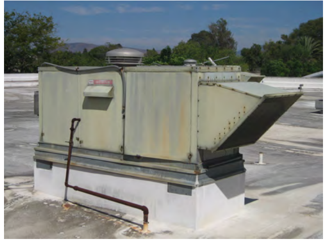
Bldg 420- Deteriorated packaged rooftop A/C units
