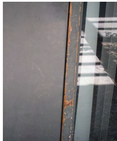
Typical exterior wood door frame finish deterioration
