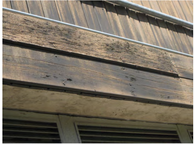
Bldg 315 - Badly deteriorated fascia/trim boards
