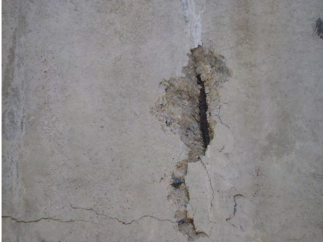
Typical concrete column spalling
