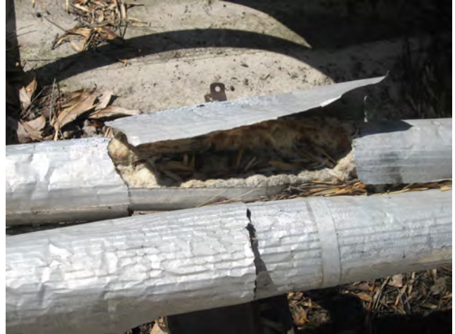
Typical deteriorated rooftop jacketed pipe insulation
