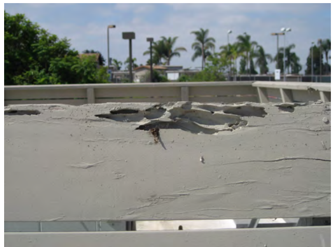
Bldg 630-660 - Typical deteriorating boards on Rooftop HVAC enclosures
