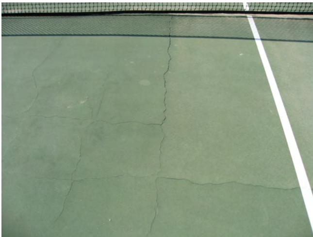
Typical tennis court surface cracks
