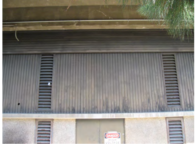
Bldg 610 - Weathered finish on exterior wood panels
