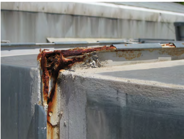
Bldg 600 - Badly rusting rooftop HVAC duct joints
