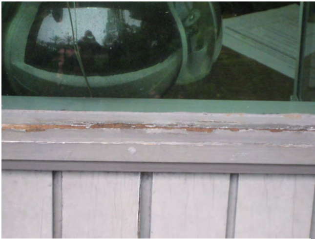
Typical exterior wood window frame finish deterioration
