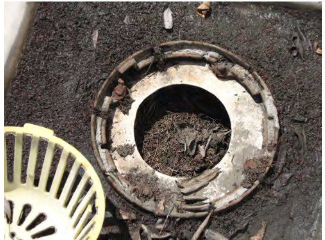
Typical clogged roof drains
