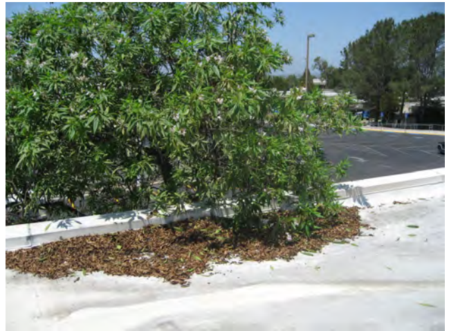
Typical tree overhang on roof
