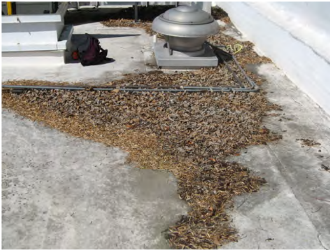
Typical roof debris build-up
