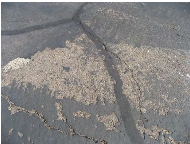
Typical parking lot paving surface wear
