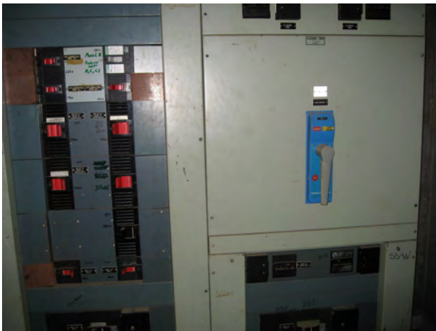
Typical old/obsolete electrical switchgear
