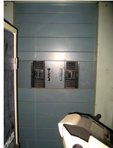
Typical old/obsolete electrical switchgear
