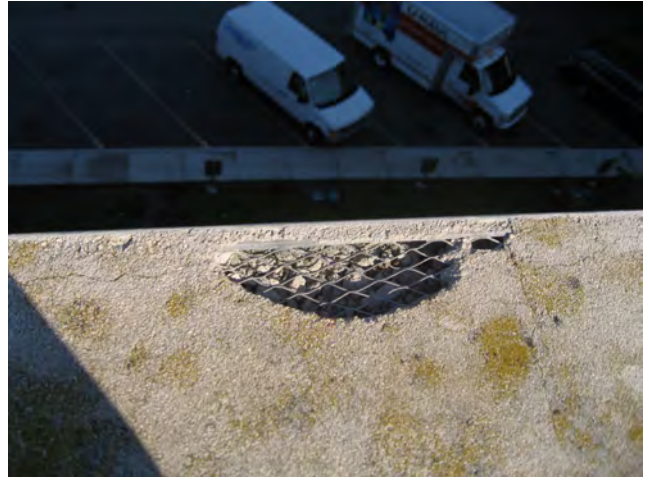
Bldg 620 - Damage on roof parapet top
