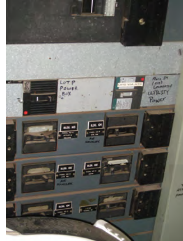
Typical old/obsolete electrical switchgear
