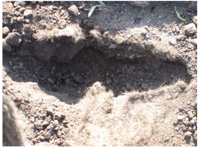
Parking lot paving deterioration-failure of old lift
