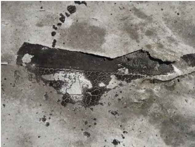
Bldg 315 - Deteriorating BUR
