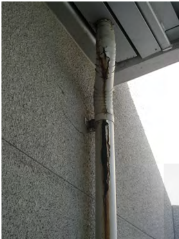
Bldg 5000 (San Ysidro) - Badly rusted/split steel downspout
