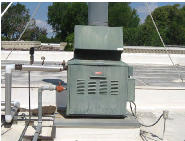
Typical deteriorating hot water boiler
