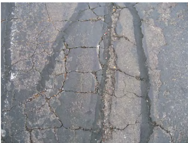
Typical parking lot paving alligating
