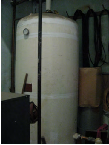
Bldg 610 - Deteriorating hot water storage tank
