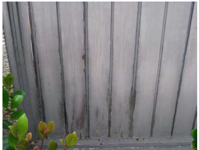
Typical exterior wood wall panel finish deterioration
