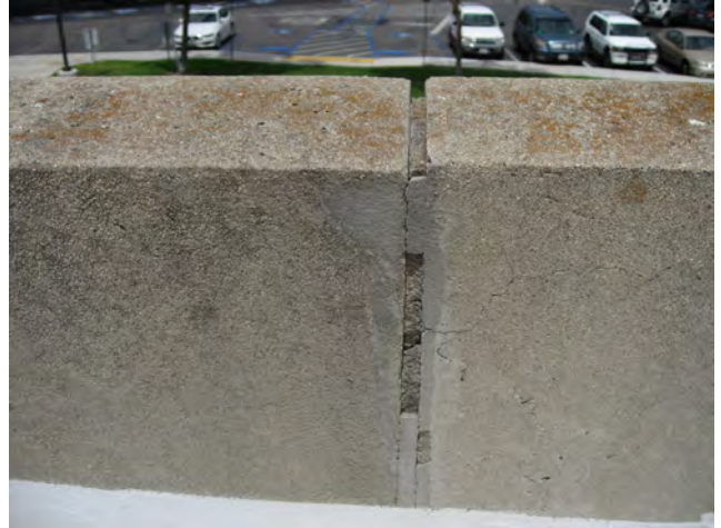
Bldg 381 - Deteriorating parapet wall joint mortar
