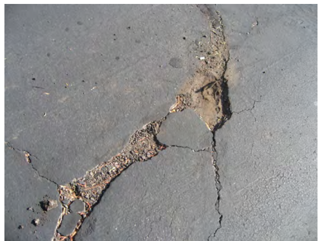
Typical failing parking lot paving wear layer
