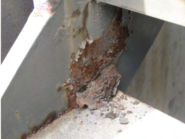
Bldg 381 - Rusting metal stringer on exterior stairway
