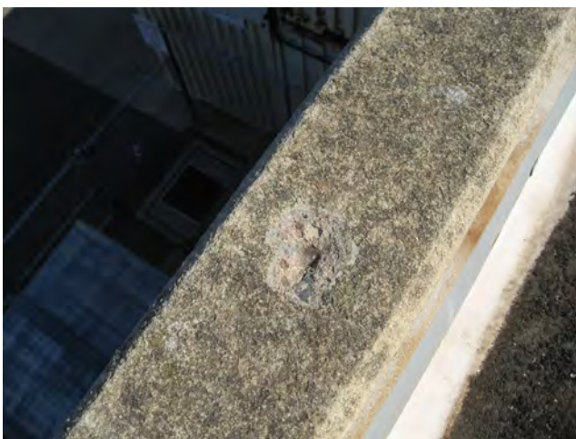
Bldg 1100 - Concrete spalling on roof parapet Exposing rebar
