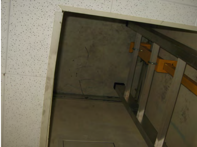
Typical failing roof hatch
