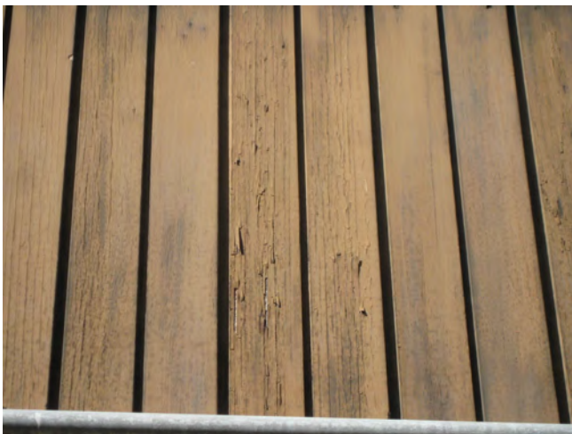
Typical exterior wood wall panel finish deterioration
