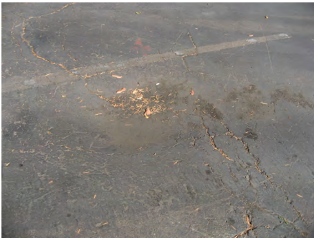
Typical parking lot paving surface crazing and hairline cracks
