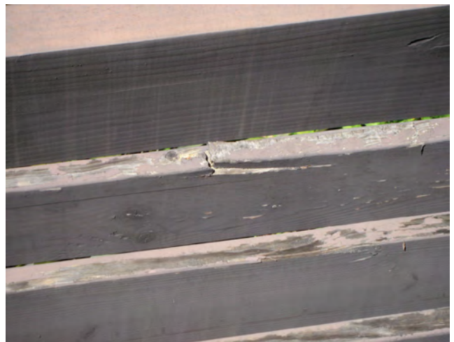
Typical deterioration on tops of sunscreen boards
