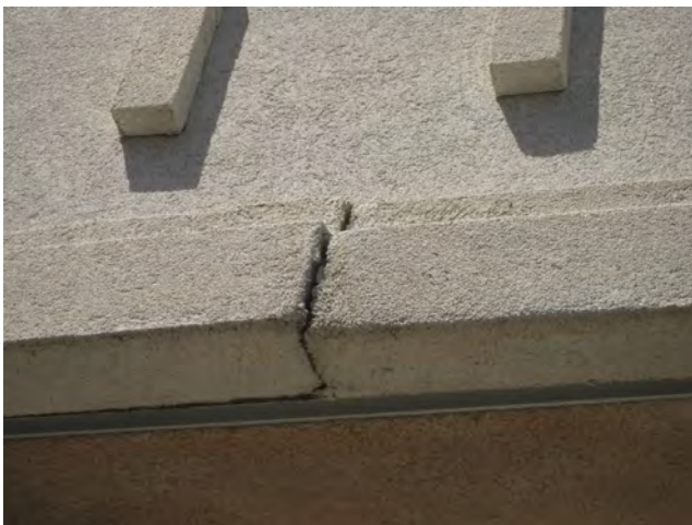
1600 Bldgs - Typical mortar deterioration at base Of roof parapets
