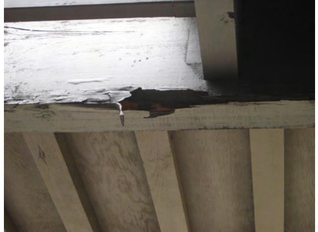
Bldg 220 - Deteriorating covered walkway roof support beam
