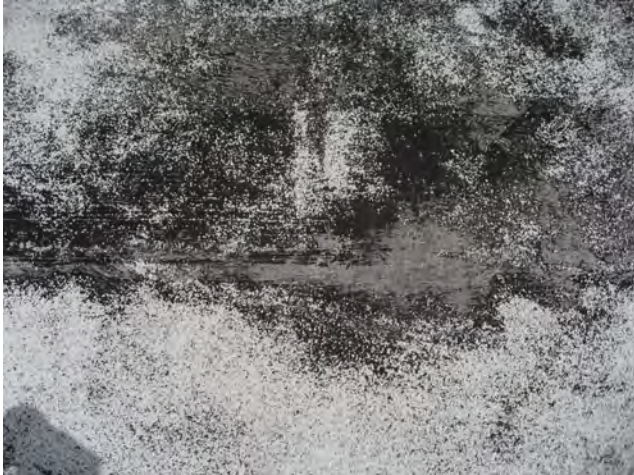
Bldg 381 - Deteriorated roof membrane
