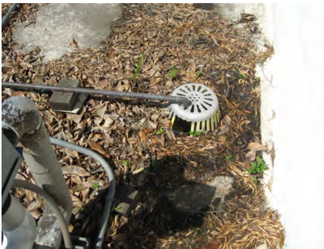
Typical clogged roof drains/sumps
