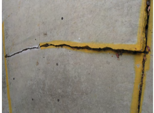
Bldg 381 - Badly cracked concrete patio area slab
