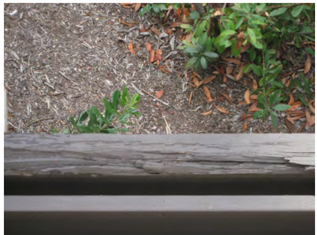
Bldg 430 - Deteriorating covered walkway roof support beam
