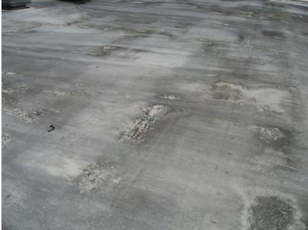
Typical dirty single-ply membrane surface
