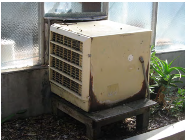
Bldg - 316 Deteriorated swamp cooler
