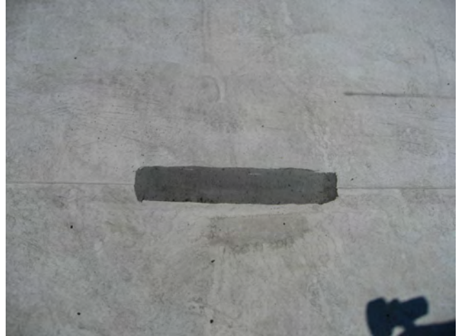
Typical roof patch on older single-ply membranes
