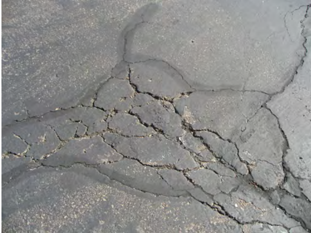
Typical larger area cracking in parking lot paving
