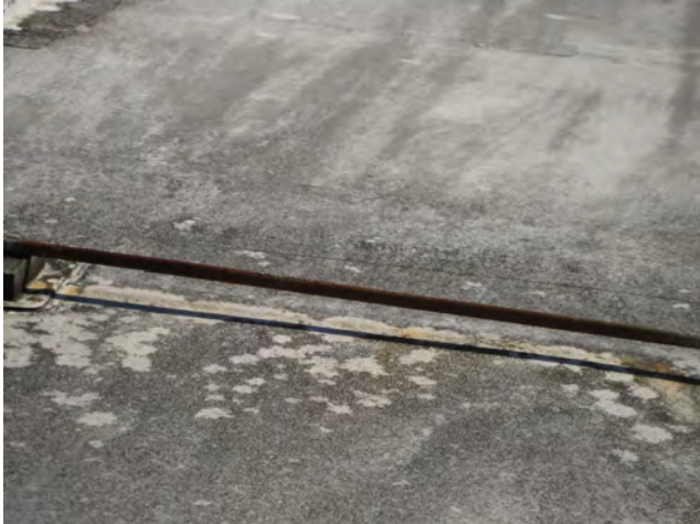
Bldg 103 - Badly rusted electrical conduit on roof
