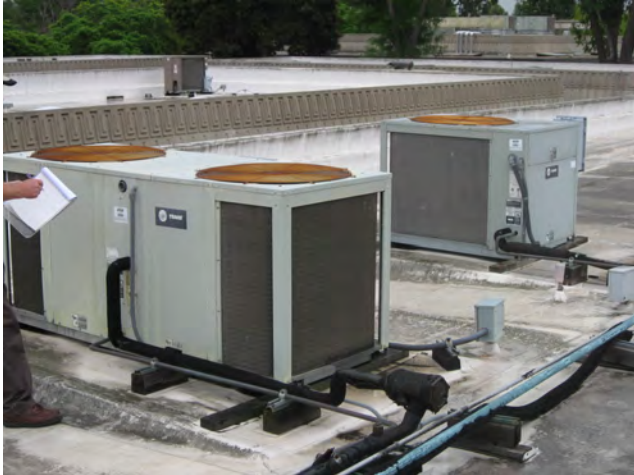
Typical older rooftop condensing units
