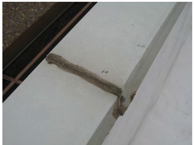
Typical deteriorating roof parapet cap joint sealant
