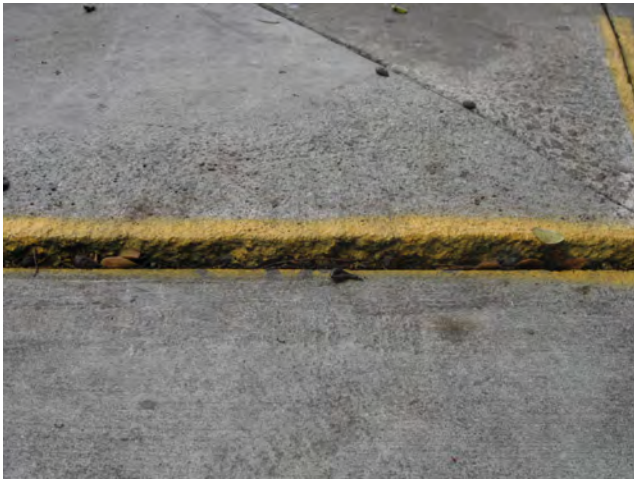
Bldg 381 - Dangerous lifting concrete walk slab
