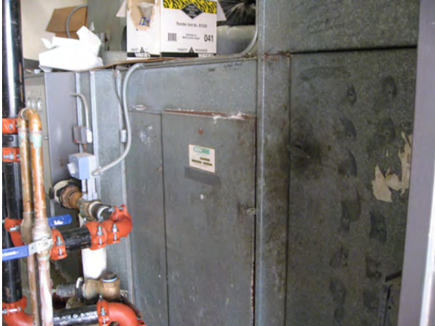
Bldg 710 - Deteriorating air handler
