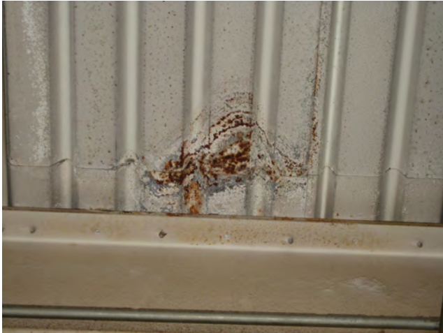
Bldg 1200 - Typical metal roof panel deterioration
