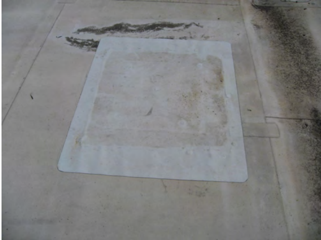
Typical roof patch on older single-ply membranes
