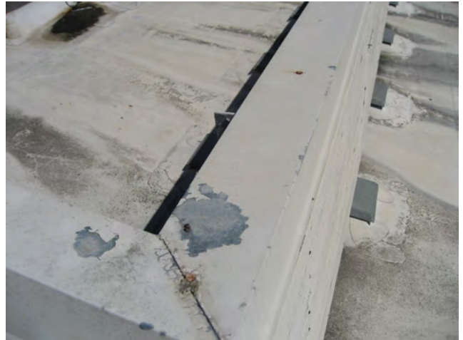
1600 Bldgs - Typical peeling paint on roof Parapet caps
