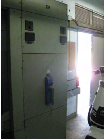
Typical old/obsolete electrical switchgear
