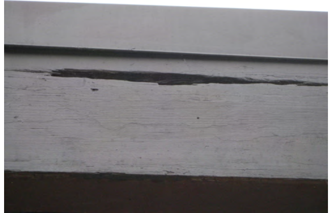
Bldg 560 - 2nd bad covered walkway wood support beam
