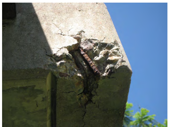
Typical concrete structural beam spalling
