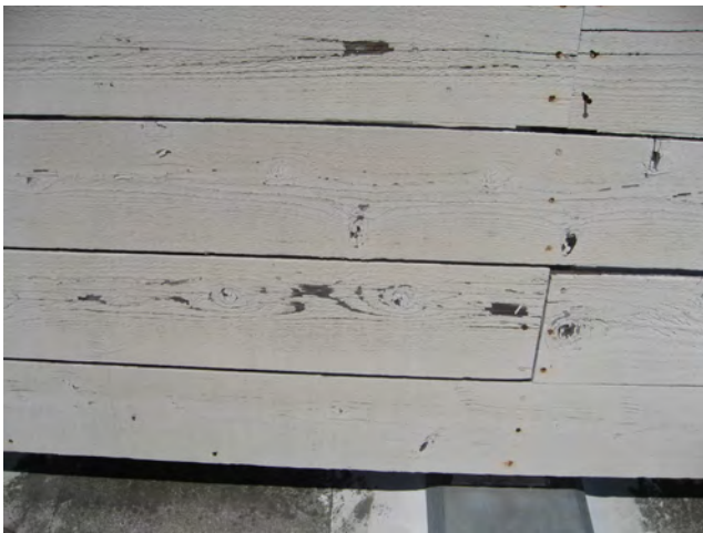
1600 Bldgs - Typical finish deterioration on rooftop HVAC enclosures
