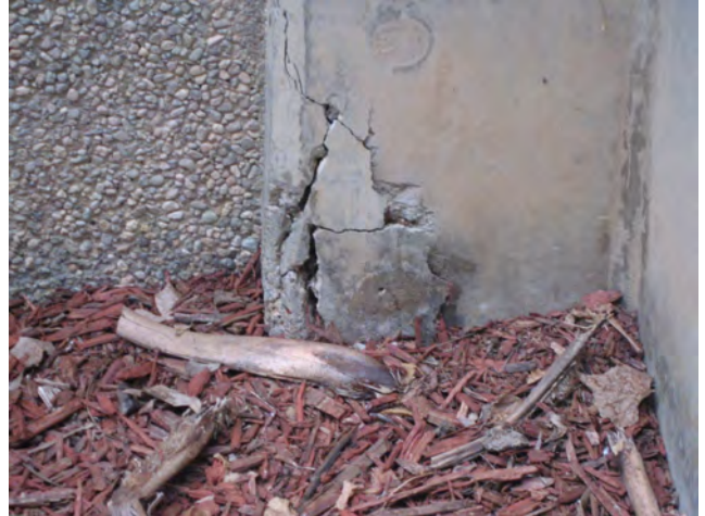
Typical concrete column spalling
