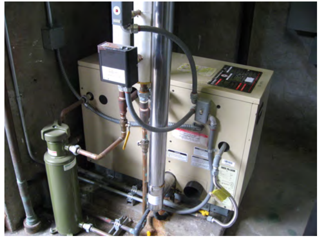
Typical deteriorating hot water boiler
