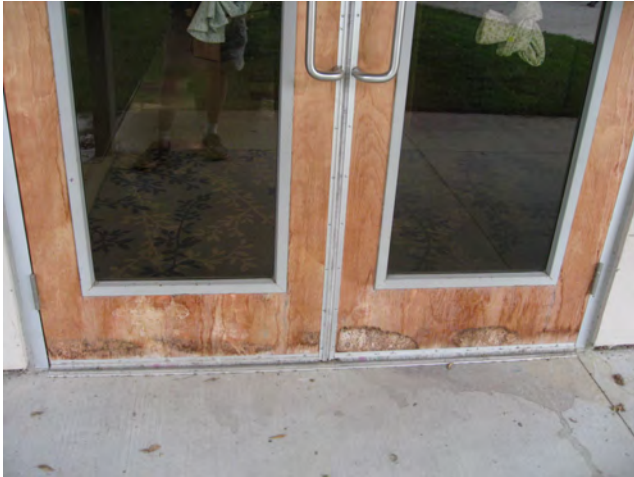
Bldg 2000 - Typical badly weathered exterior Door finish
