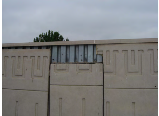
Bldg 2000 - Typical EIFS damage on rooftop HVAC enclosures
