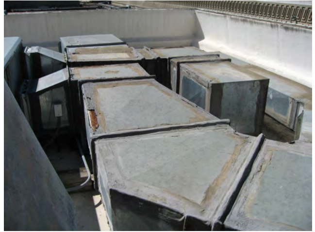
Typical deteriorating rooftop ductwork Seam sealant
