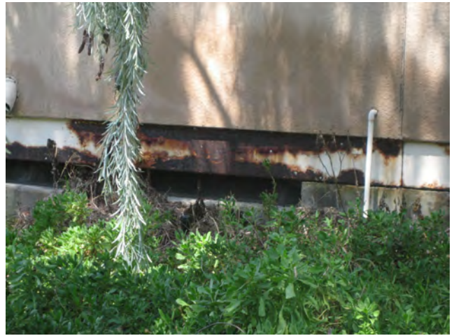
1600 Bldgs – Typical rusting on metal at base of buildings
