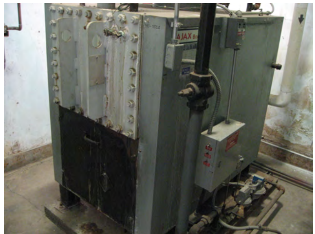
Bldg 610 - Deteriorating hot water boiler
