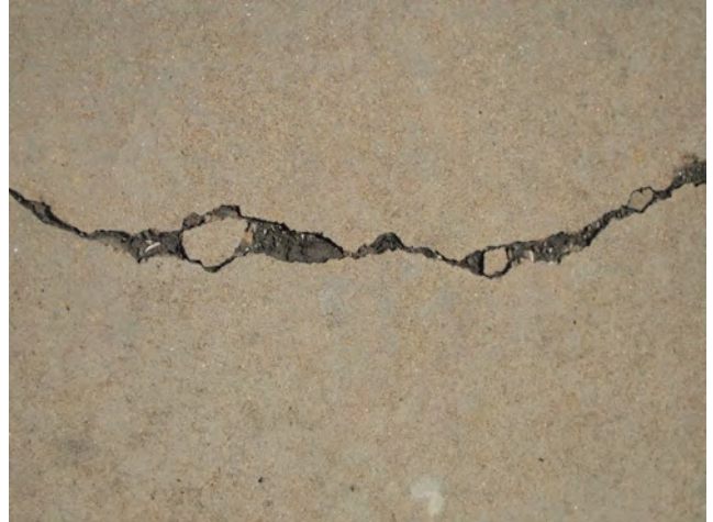
Typical concrete walkway cracks
