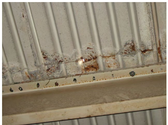
Bldg 1200 - Typical metal roof panel deterioration
