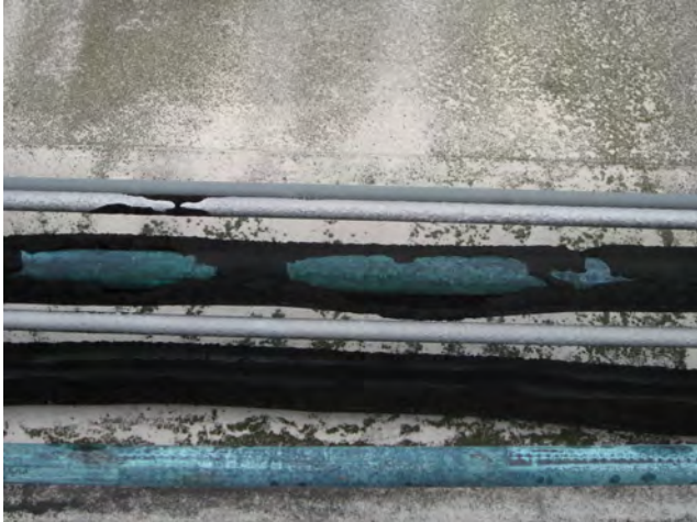
Typical deteriorated rooftop foam pipe insulation
