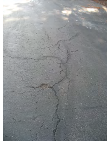
Typical smaller cracks in parking lot paving
