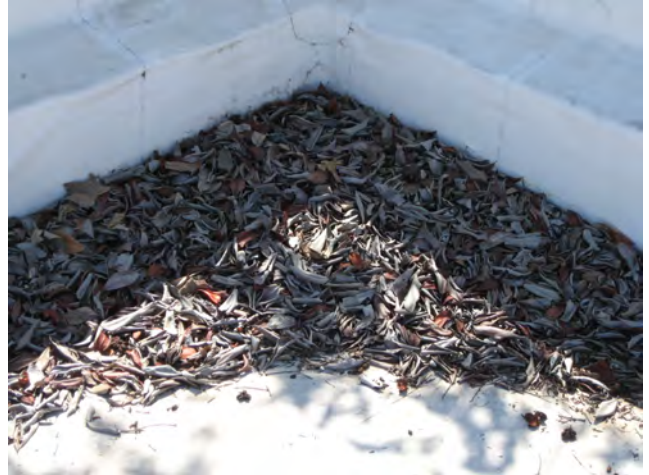
Typical roof debris build-up
