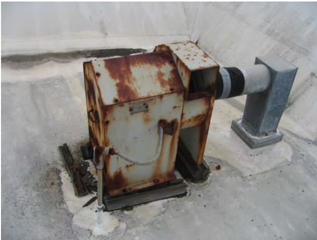
Bldg 590 - Badly deteriorated rooftop exhaust fan
