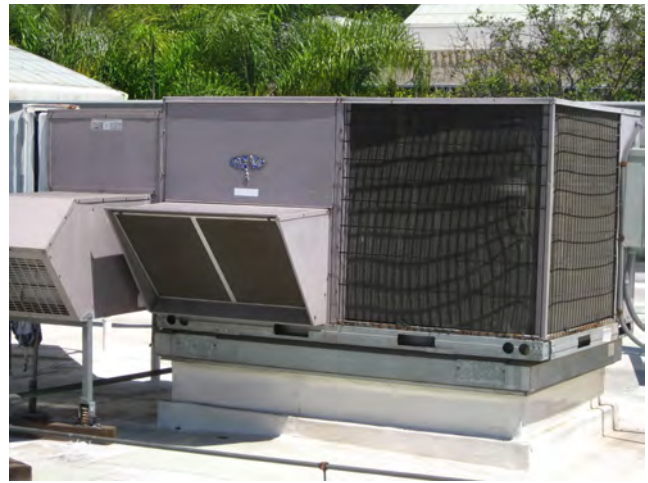
Typical older rooftop HVAC units w gaspaks
