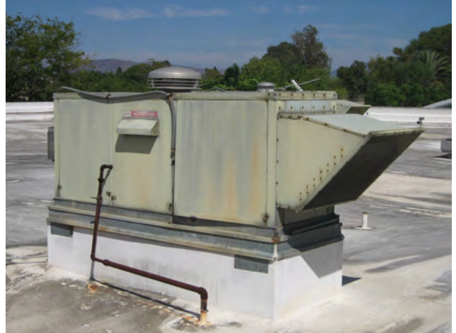
Typical older rooftop packaged HVAC units
