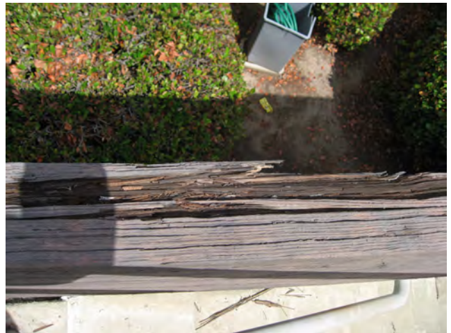
Bldg 381 - 2nd badly deteriorated walkway roof support beam
