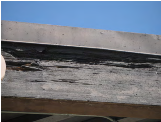
Bldg 750 - Badly deteriorated covered walkway Roof beam
