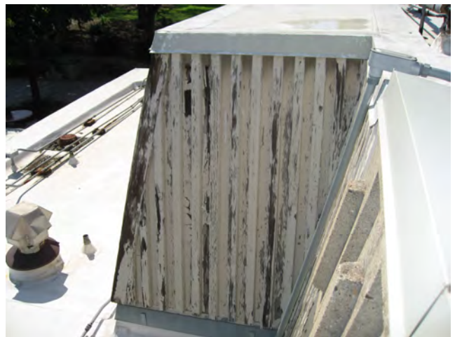
Bldg 340 - Deteriorated wood parapet
