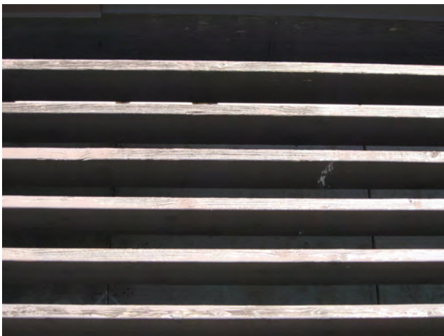
Typical deterioration on tops of sunscreen boards
