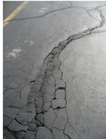
Parking lot paving slumping
