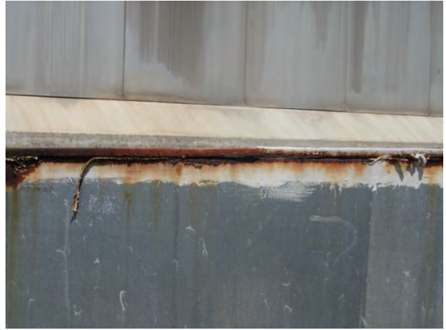
Bldg 600 – Badly rusting rooftop HVAC duct seams
