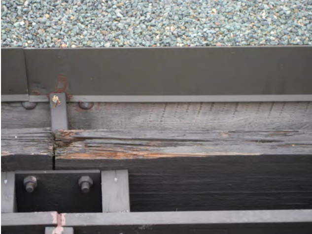
Bldg 560 - Deteriorating covered walkway wood support beam
