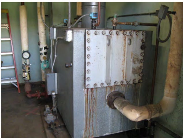
Typical aging/deteriorating boiler
