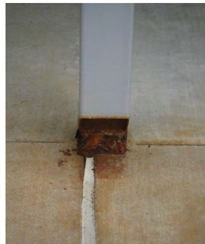
Bldg 2000 - Typical rusting of base of steel walkway Roof support columns
