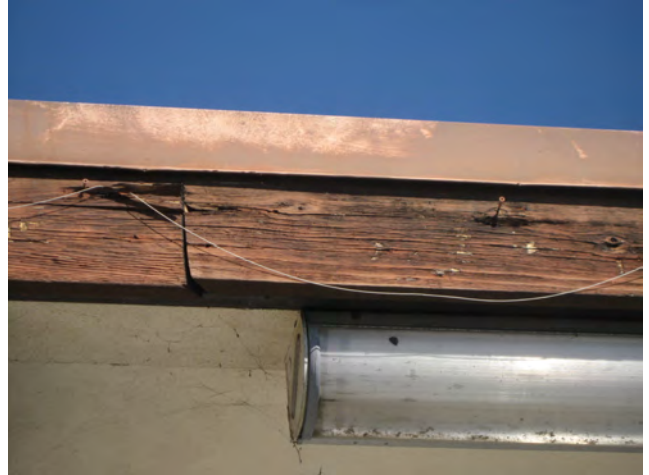
Bldg 750 - Badly deteriorated wood roof fascia
