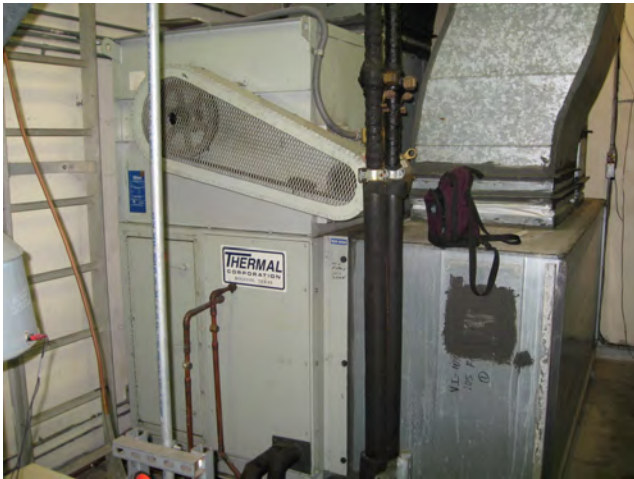
Typical air handler in mechanical room
