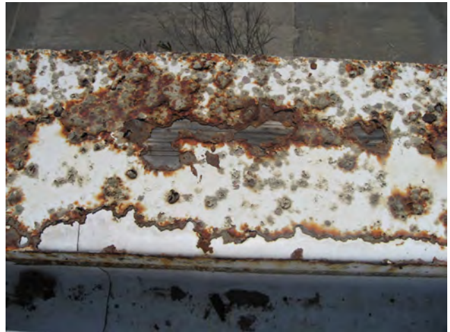
Bldg 9000 (Crown Cove) – Typical totally deteriorated metal parapet cap flashing
