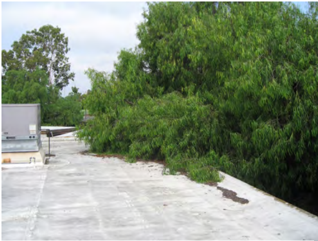
Typical tree overhang on roof
