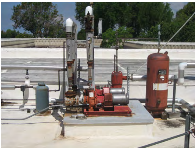
Bldg - 430 Deteriorated rooftop gas boiler and Circulating pumps
