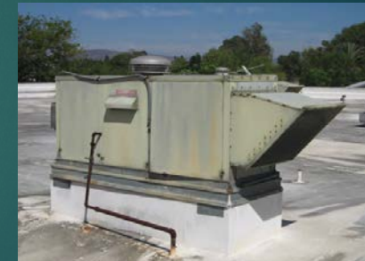
Typical Deteriorating Rooftop HVAC Units
