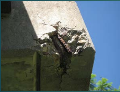
Typical Spalling on Structural Beams and Columns
