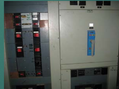
Typical Obsolete Electrical Switchgear
