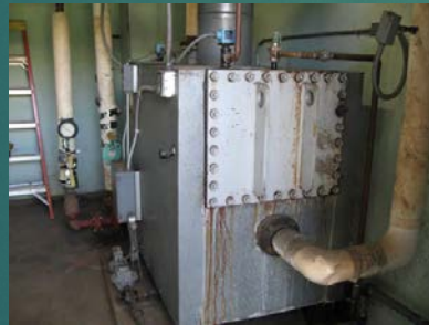
Typical Deteriorating Hot Water Boilers
