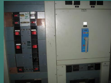
Typical Obsolete Electrical Switchgear
