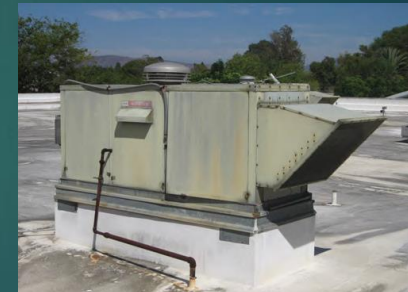
Typical Deteriorating Rooftop HVAC Units
