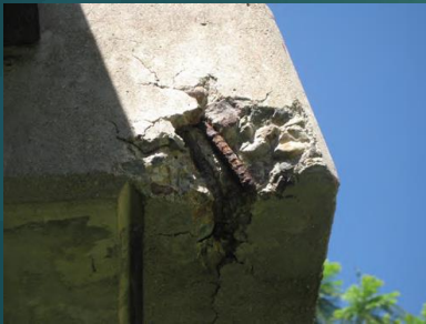
Typical Spalling on Structural Beams and Columns
