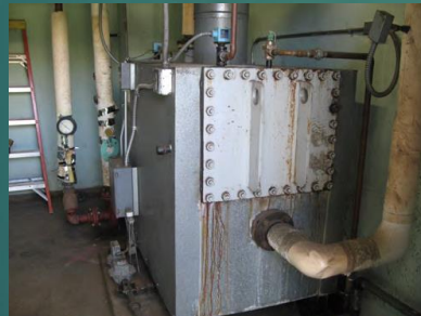
Typical Deteriorating Hot Water Boilers
